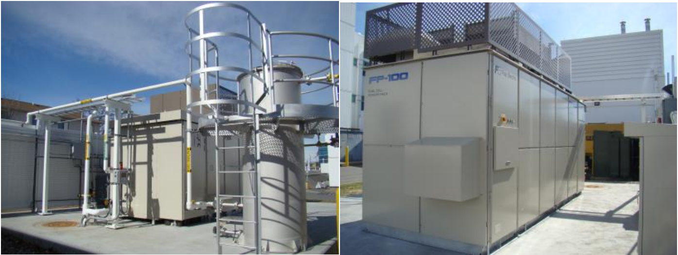
SUNY Poly's fuel cell operating in parallel with the on-site emergency generator.
